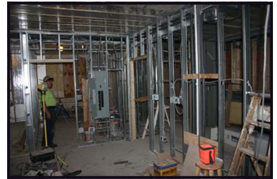
ABOVE: Priory interior, looking from the dining room to one of the bedrooms and the kitchen.
