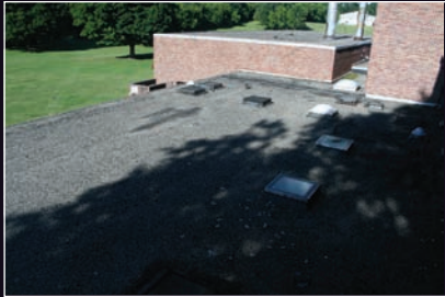
ABOVE: Our 50-year-old roof is dying and needs replacing.
